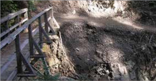
2012 storm event damage resulted in closure of part of the Bootjack Trail.
