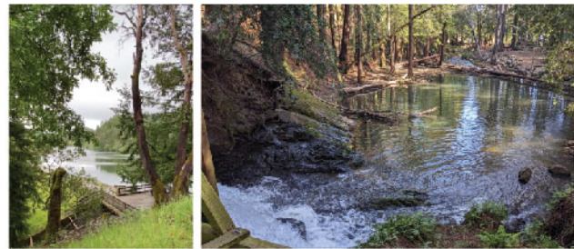
Wooden deck at the top of the spillway at Lake Lagunitas (left), bottom of the spillway next to picnic area (right)
